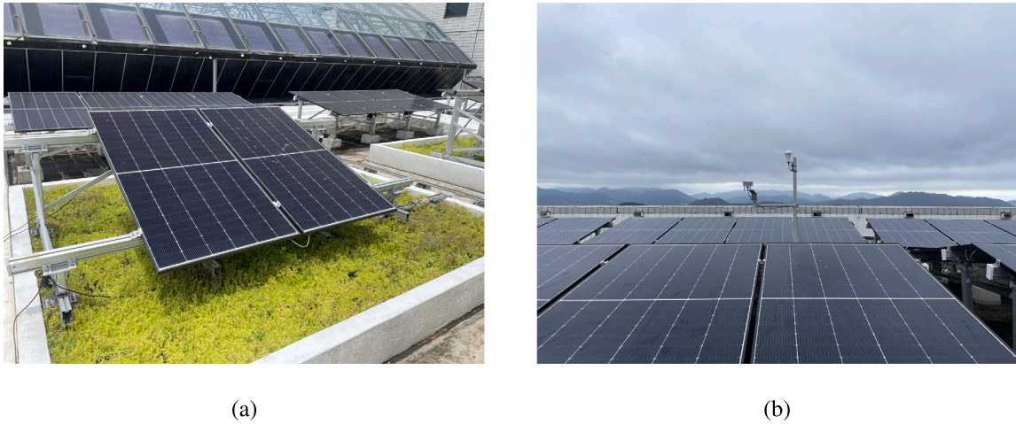
Fig. 1. The selected experimental sites. (a) PVIGR; (b) Concrete rooftop PV system (RPV).
