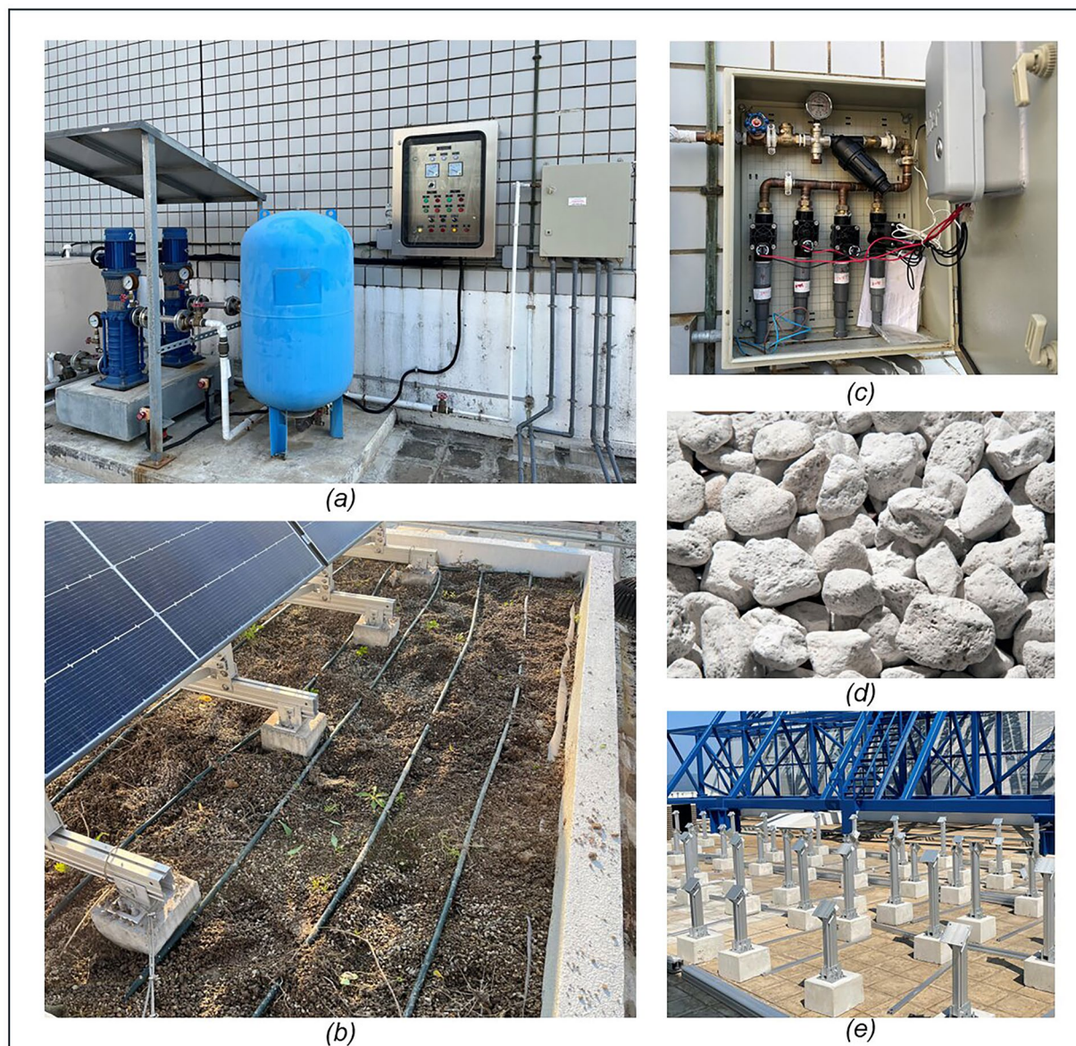
Fig. 3 (a) Automated integration system, (b) Drip irrigation pipes placed on soil, (c) Control panel of the irrigation system, (d) Concrete plinths and (e) Connected PV mounting frame.
